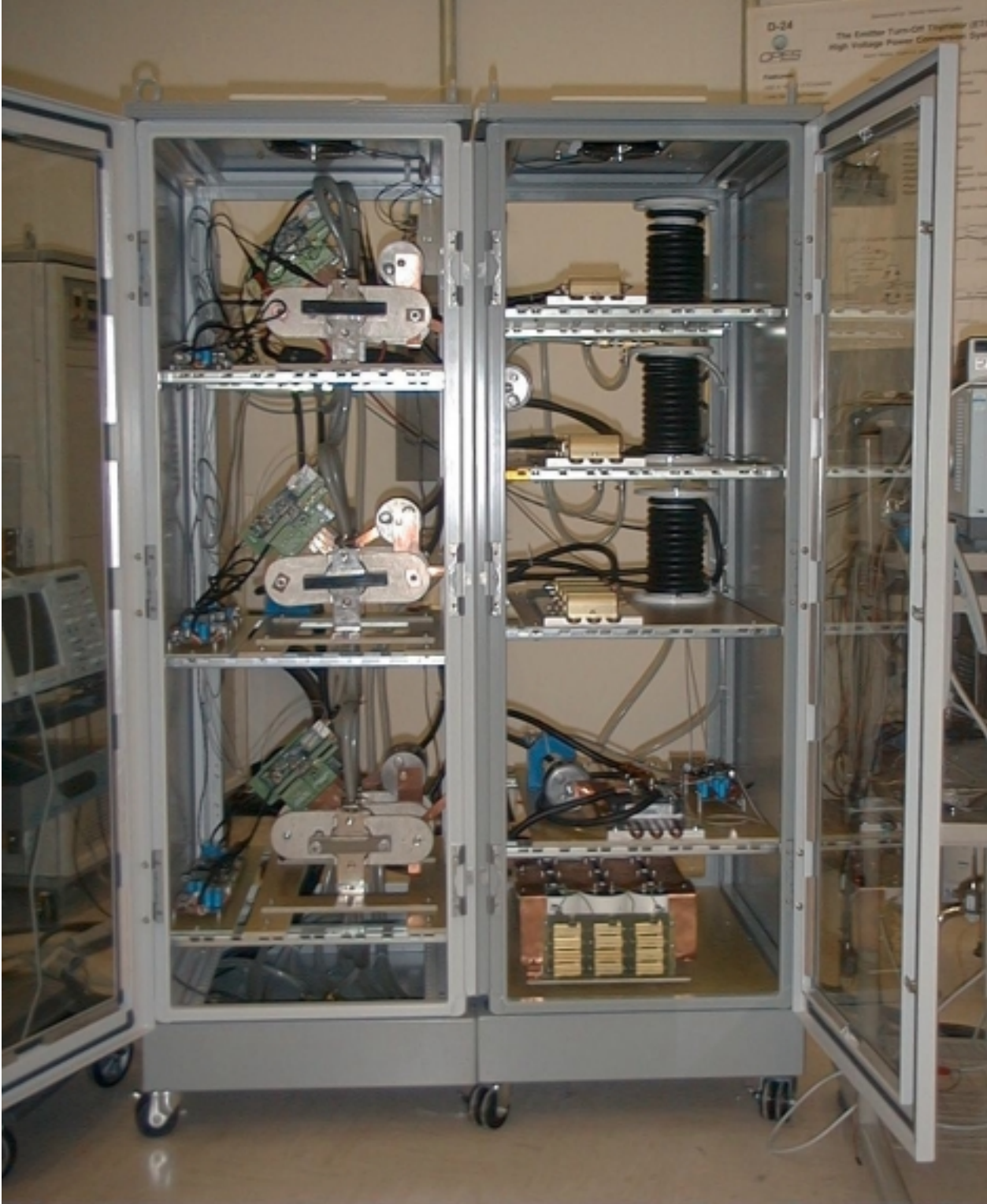
Figure 38: Picture of the ETO-based inverter
