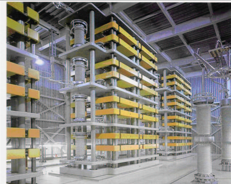
Thyristor Valves: 300 MW, 250 kV, 1200A, 6kV, 2500 A LTT (Toshiba), 1992
